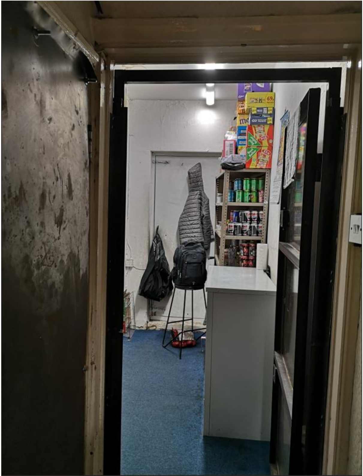
Diamond Food & Wine – sealed fire exit 27/02/26
